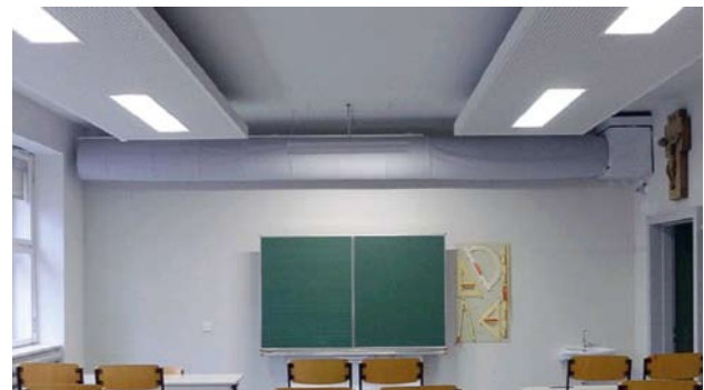
Figure 6. Active overflow ventilation in prototype classroom in Innsbruck, air inlet via textile diffuser and fan from corridor (preheated supply air from central heat recovery unit at the attic without duct via staircase and corridor).
