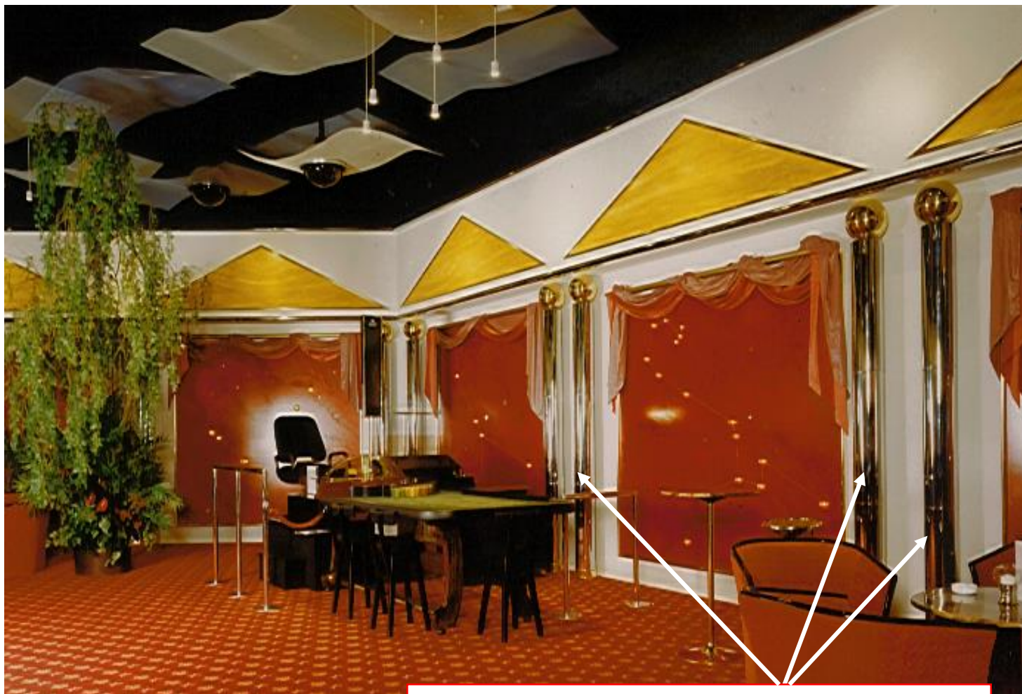
Air diffusers behind columns
