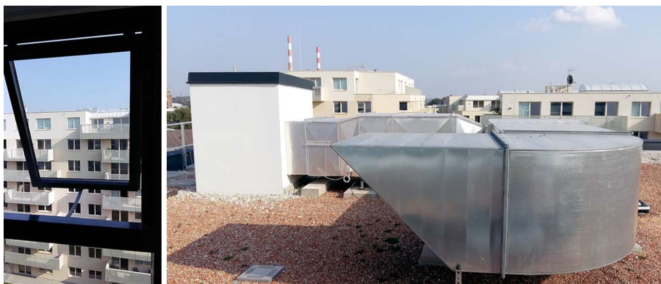
Figure 2. Air inlet window with chain actuator (left) Exhaust ventilator on roof (right).
