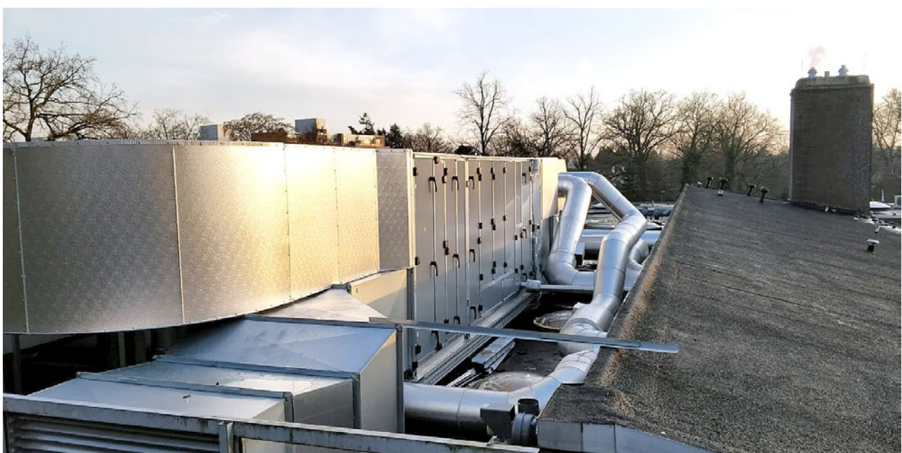
Figure 1. SchoolVent air handling unit with insulated ducting.
