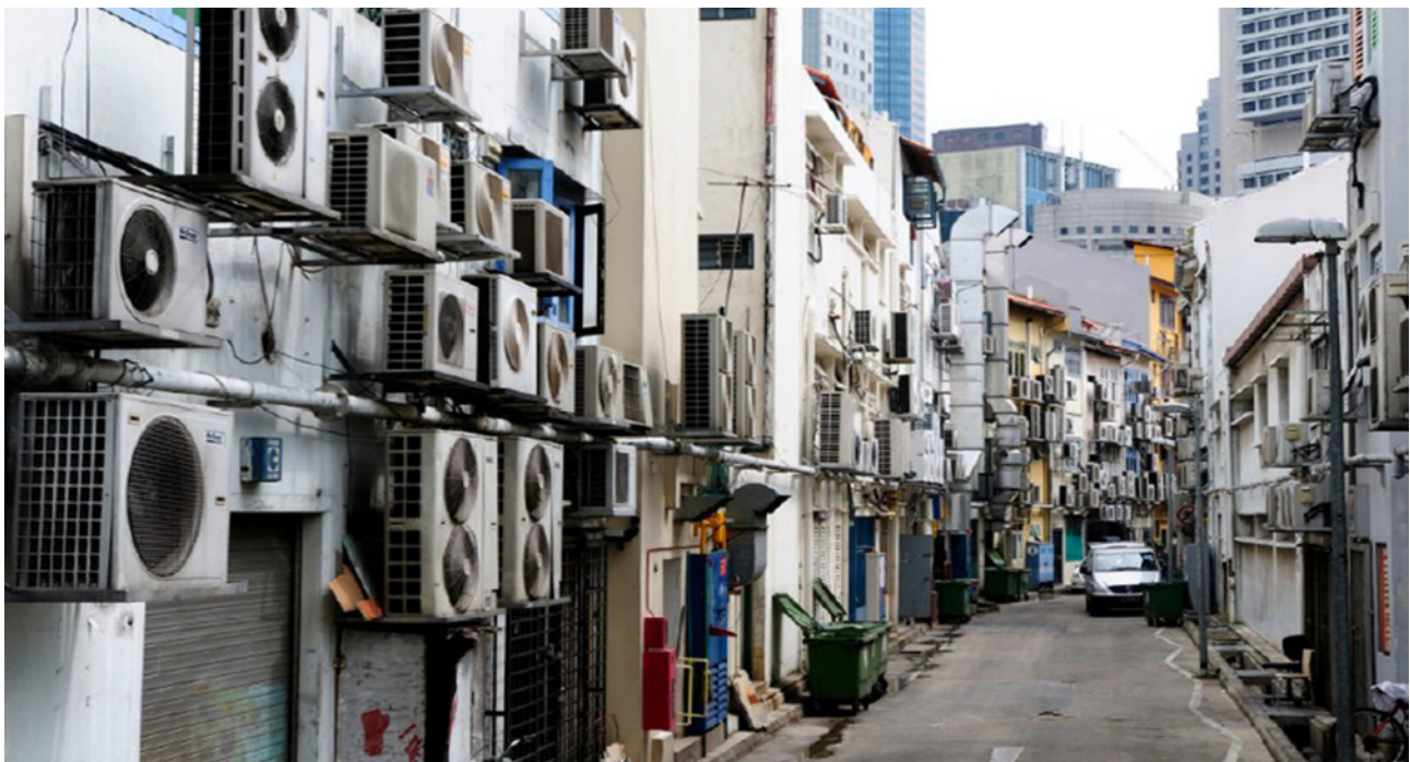
Figure 2. Space cooling during Summer - Typical sight in areas with high occurrence of split air conditioning systems.
