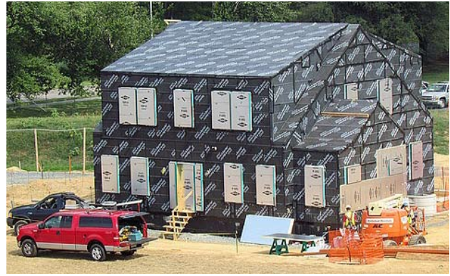
Figure 1. NZERTF prepared for a quality control airtightness test (Note that windows openings are covered to measure tightness of only the opaque portions of the building envelope).
