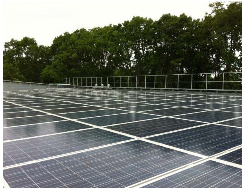
Figure 2. Photovoltaics installed on the roof of the retirement home in the passive house area Vallda Heberg [6].
