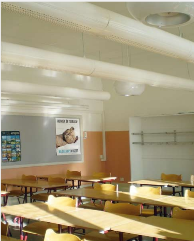
Figure 1. High velocity terminals installed in a class room.
