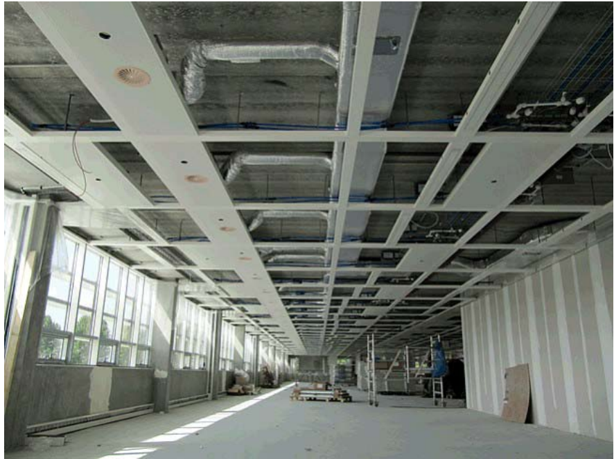
Figure 4. Ceiling of concrete core activation for heating and cooling, with integrated air diffusers in the ceiling panels..
