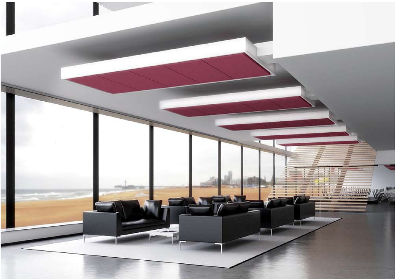
Figure 1. The chilled beams integrated with radiant panels (red colouring).
