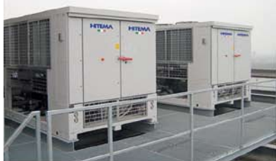
Inverter Technology Compressors - Total Load 3,2 Mw
