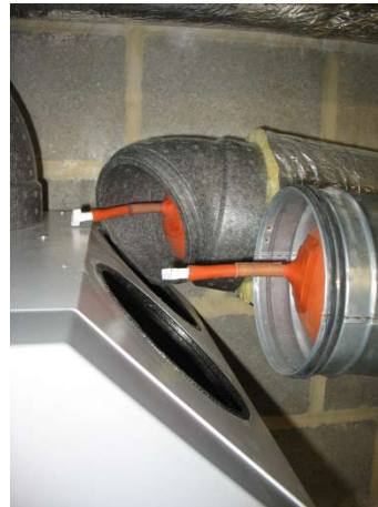
Figure 3. Sealing the main ducts just before or after the air handling unit is an option, but it generally requires dismantling the ducts.
