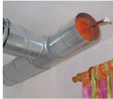
Figure 2. Rubber bladders can be useful for sealing ventilation ducts.
