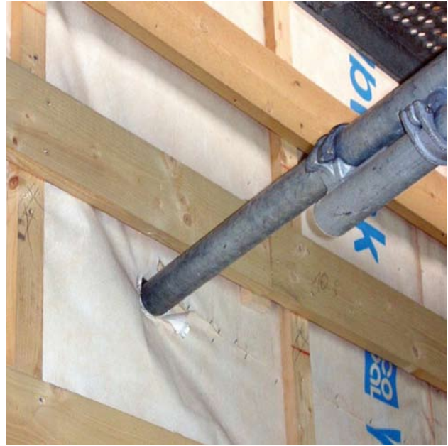
Figure 2b. Leaky wind barrier detail, from anchoring of the outside scaffolding (Photos: Tormod Aurlien).
