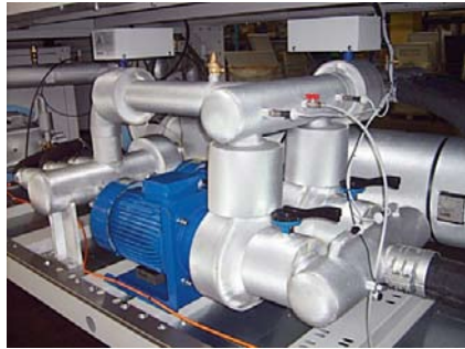
Figure 6. Inverter driven double pump.
