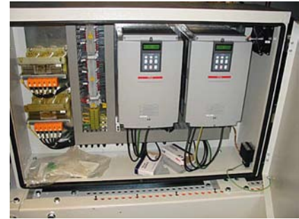
Figure 7. Electrical board with inverters for pumps.
