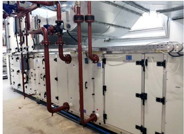
Figure 3. Air handling unit in the facility in installation phase.
