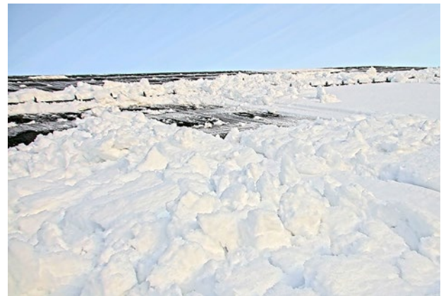
Figure 3. Example of daily photographic inspection to evaluate snow coverage on the roof (Dec 15th to Jan 14th).
