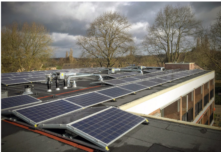
Figure 1. Solar panels on the roof of De Benring building.
