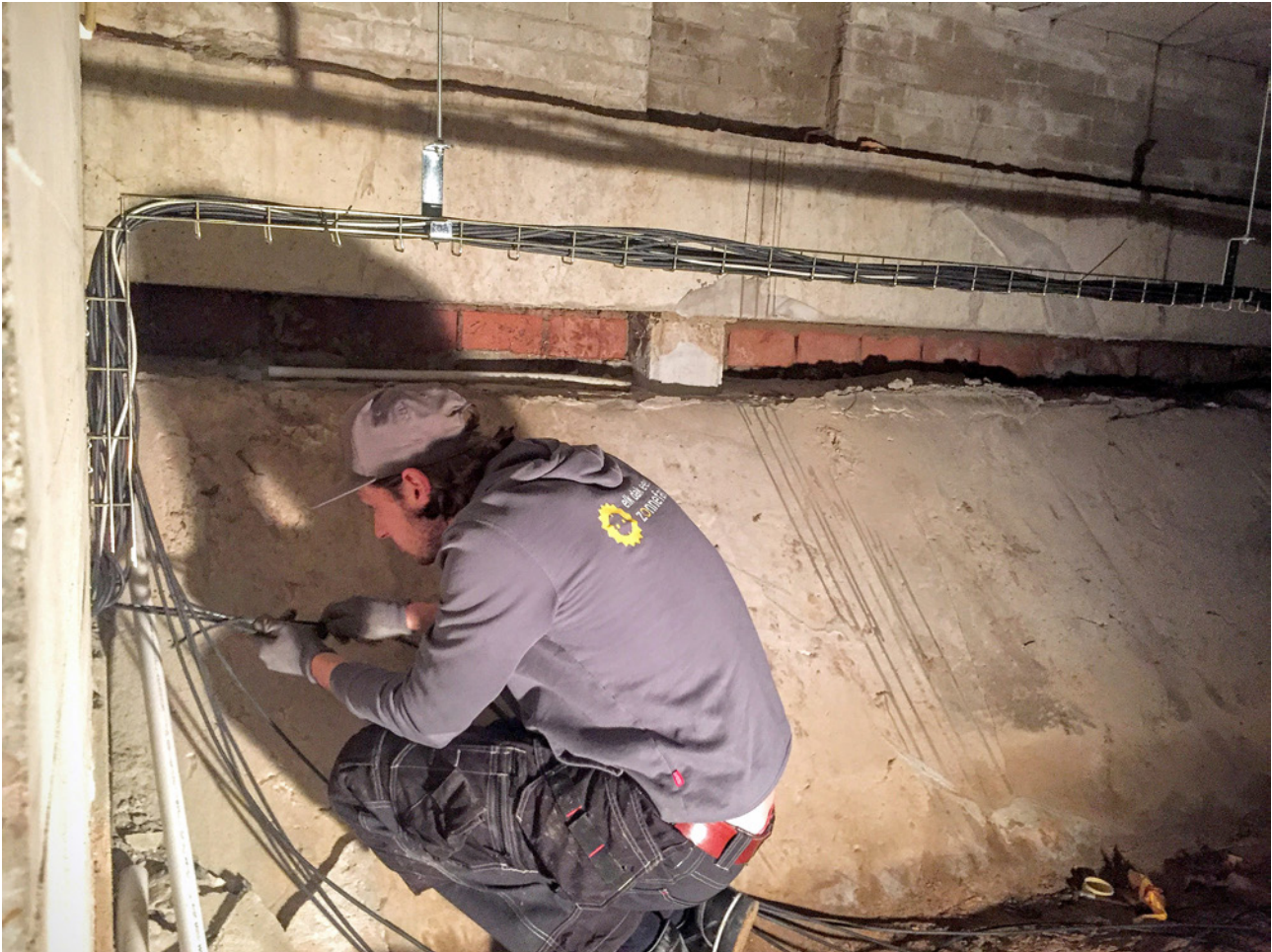
Figure 2. Installing solar panels in existing building, requires installers to improve electrical infrastructure.
