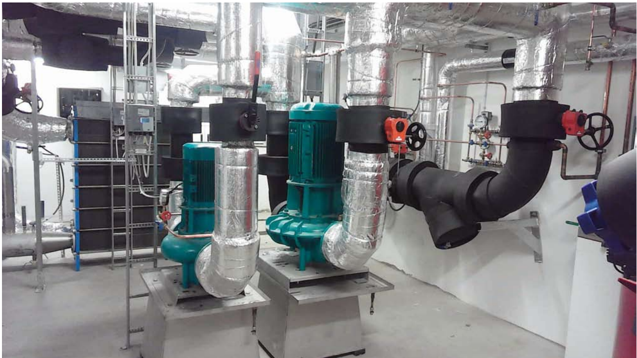
Figure 3. The main circulation pumps for the Skanska Deep Green Cooling in the front and the ground heat exchanger in the rear.
