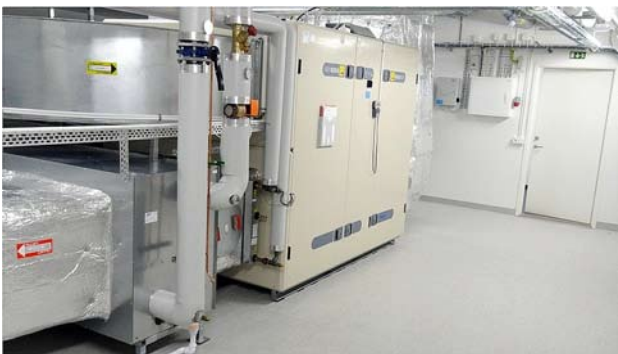
Figure 2. The AHU in southern building body, LA1, with supply air duct in the bottom left of the picture with heating coil closest to the ventilation unit and then cooling coil. LA2 in the northern building body is similar.
