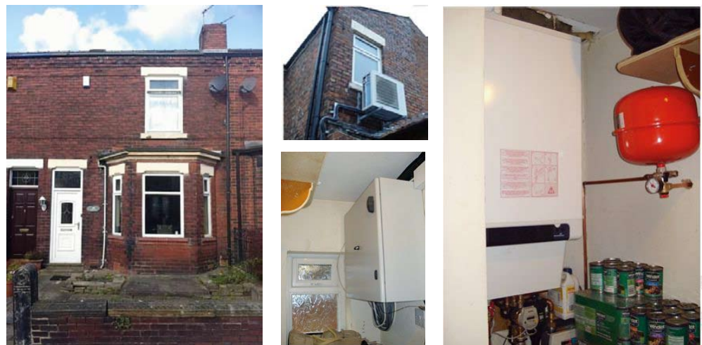
Figure 4. The HYBRID heat-pump system was tested in this 110 year old, terraced UK house during winter 2011-12. A family of three lived in the building with heated floor area of 140 m 2 . The house was heated with hot water radiator system with design supply temperature of water 70°C in design outdoor temperature of -6°C.
