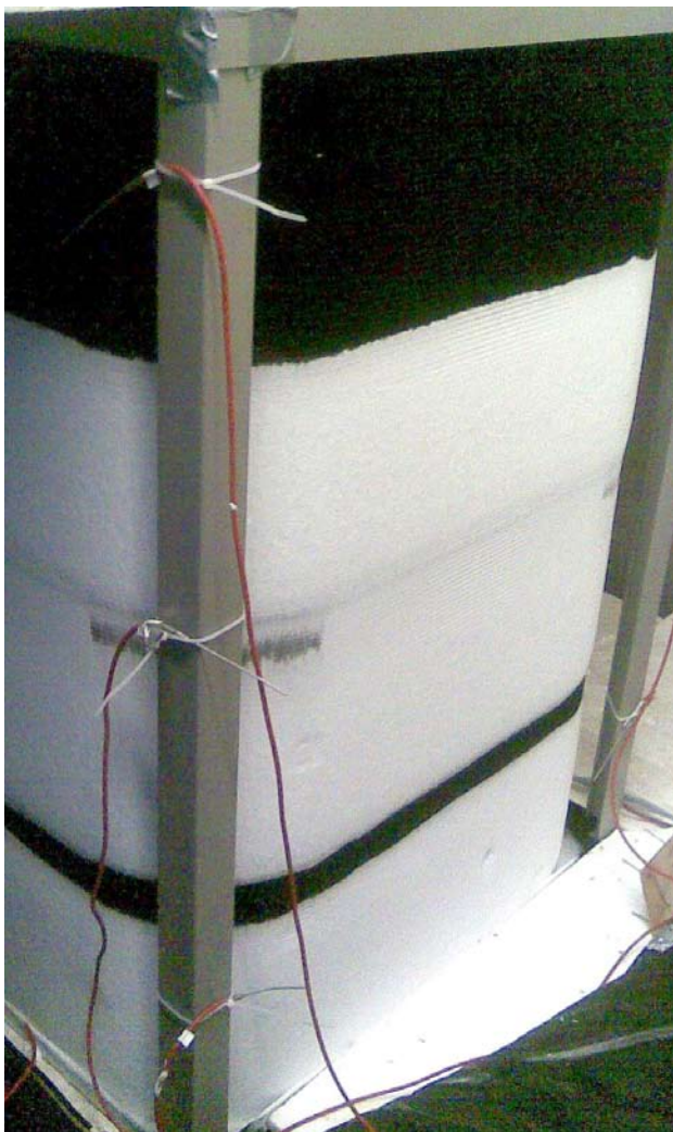
Figure 2. Ice build-up on an evaporator.
