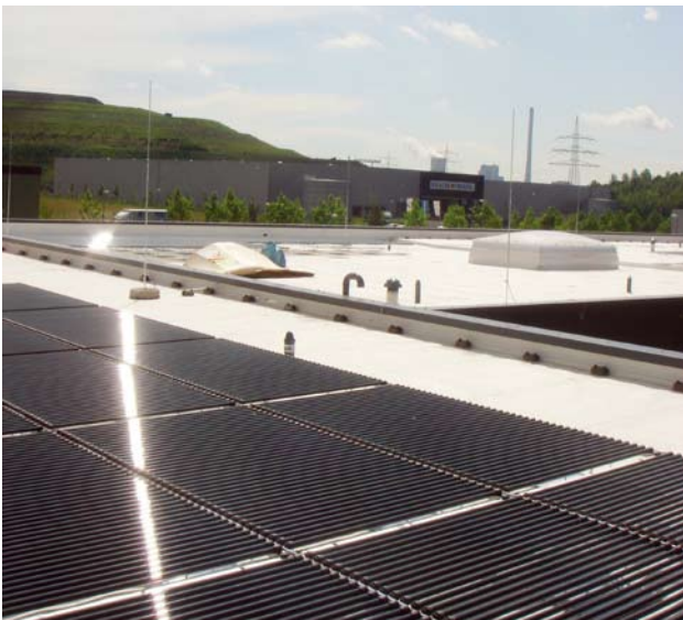
Figure 3. View on the roof with photovoltaic panels and standard white roof coating.
