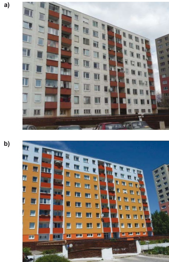
Figure 1. Front side (south facade) of the building. a) before renovation, b) after renovation.
