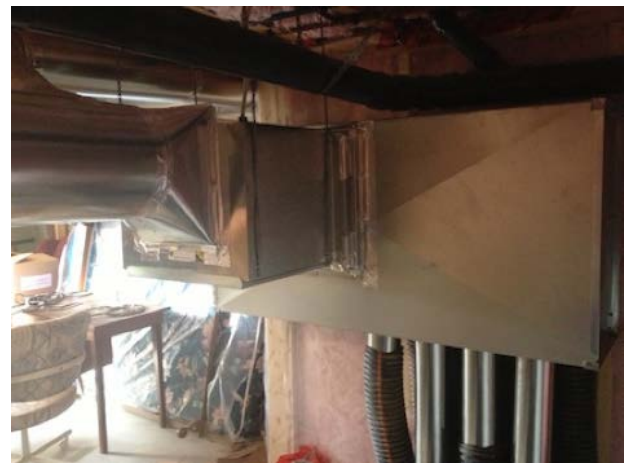
Figure 8. Ductwork header connected to earth tubes and fan unit.
