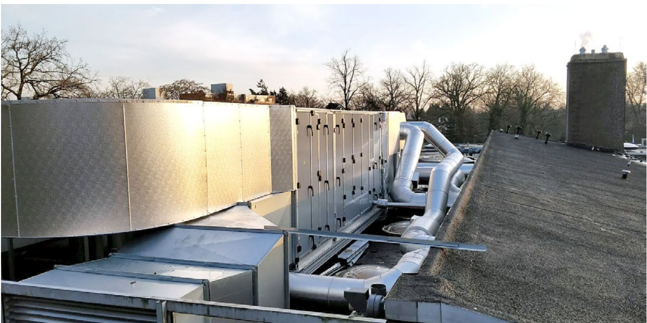
Figure 1. SchoolVent air handling unit with insulated ducting.
